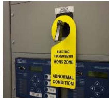
Use of Flagging Hanger “Abnormal Condition”
