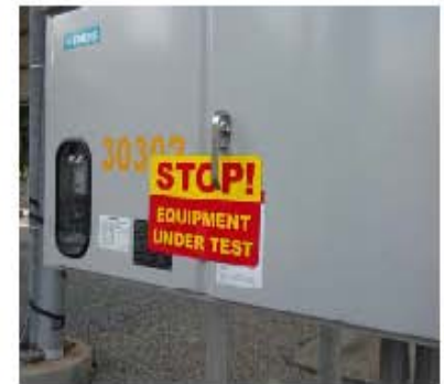
Use of “STOP - Equipment Under Test” Magnet
